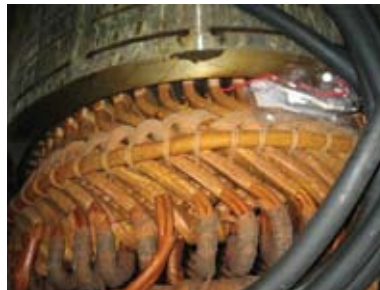
End turn bracing
