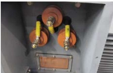
Conduit box with standoff insulators
