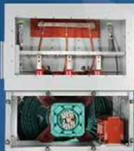
High Voltage with Rear Cover Removed
